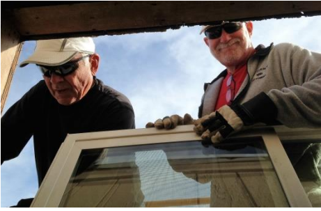
Bob Westbrook and Peter Wiley installing one of the new windows in the annex.
